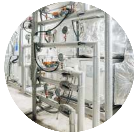
The latest water supply and sewerage system
