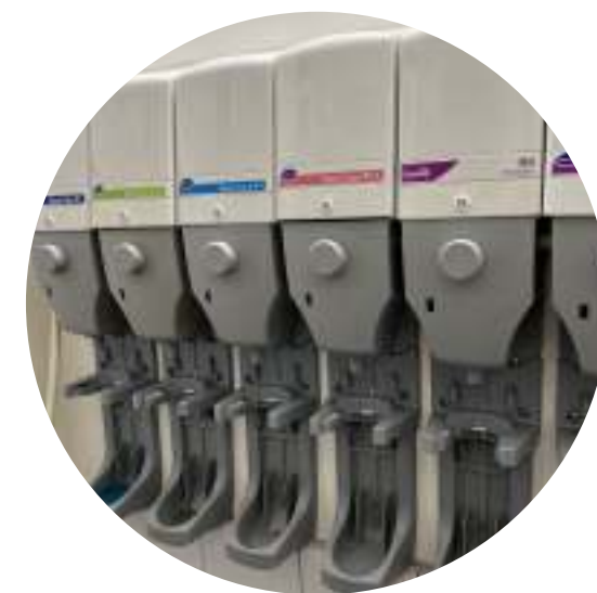
Hot water circulation system, own laundry room
